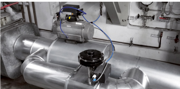
3. "DE" Station, Line 6 supply flow BSV DN 200
