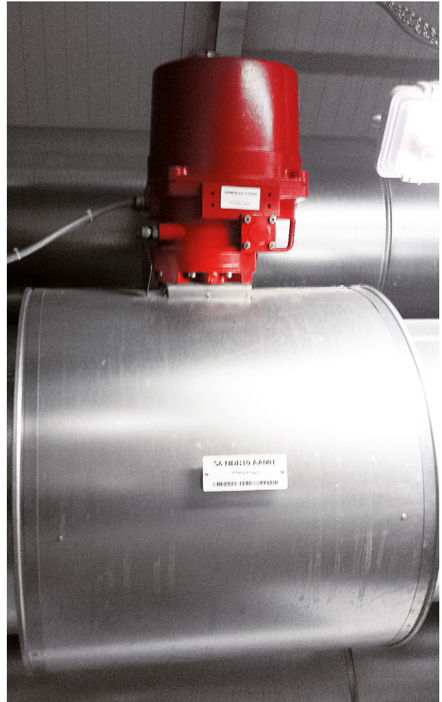
5. "HKW" line 6 return flow BSV with motor drive DN 250
